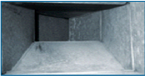
A duct after cleaning.
